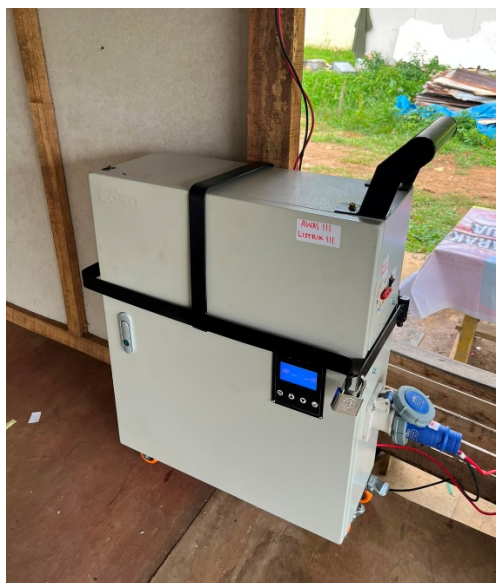
Figure 1. Portable PV power station
